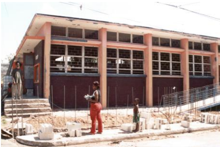
The building at 3 Albert Street housing the ceramic production unit being renovated
